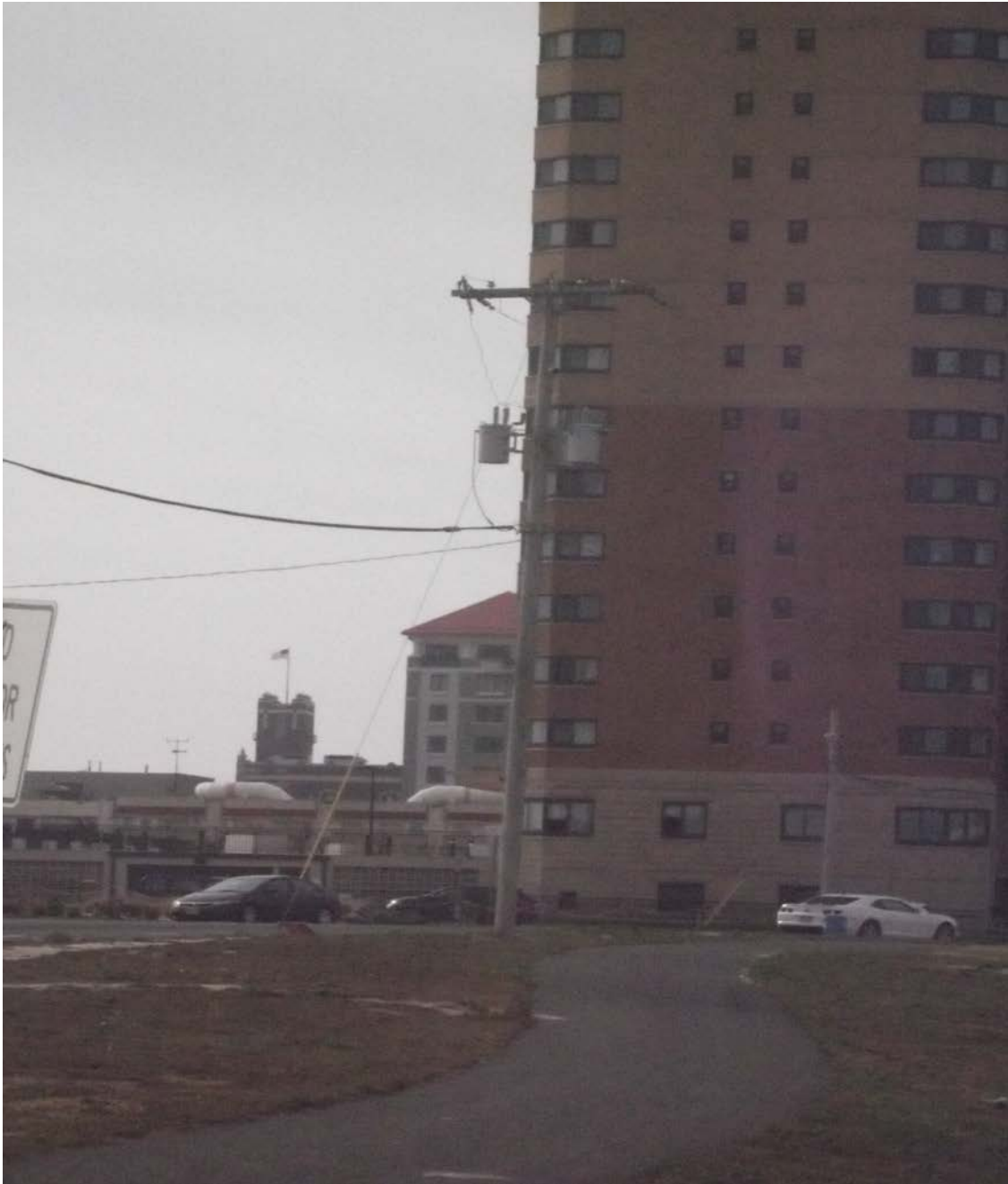
Existing JCP&L Pole Mounted Transformer for New Underground Service
