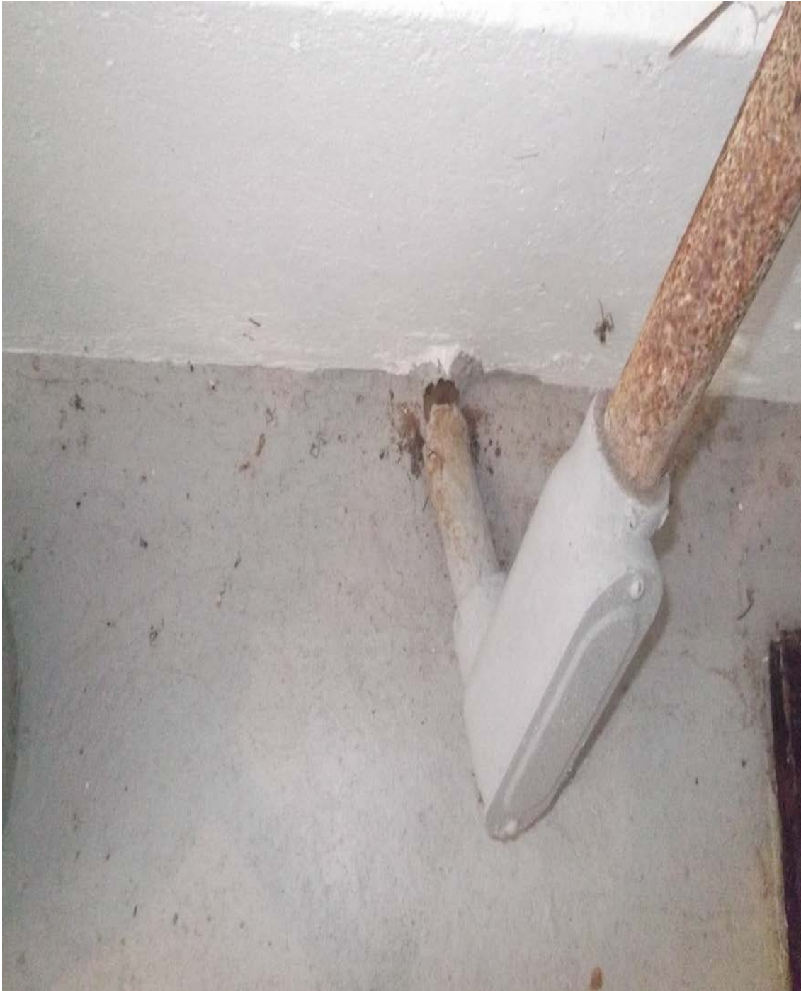
Existing Damaged Underground Service to be Removed & Replaced
