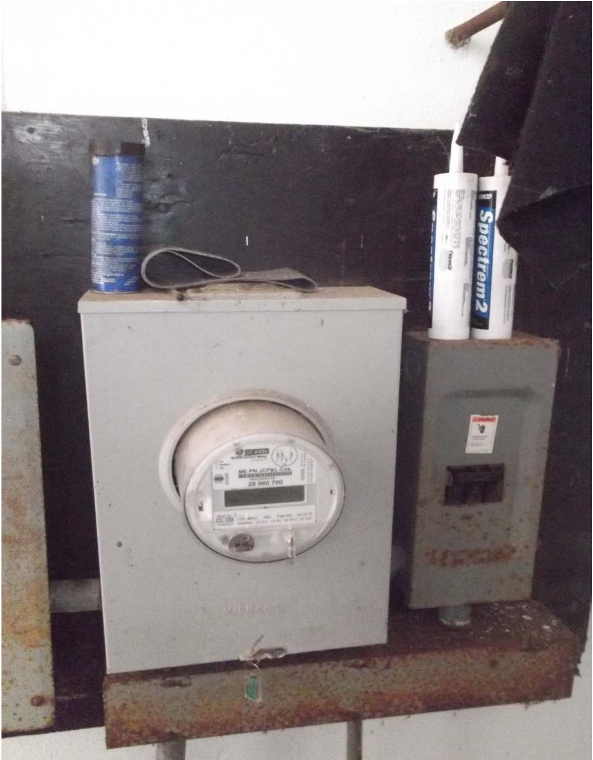
Existing JCP&L Meter & Main Circuit Breaker to be Removed & Replaced
