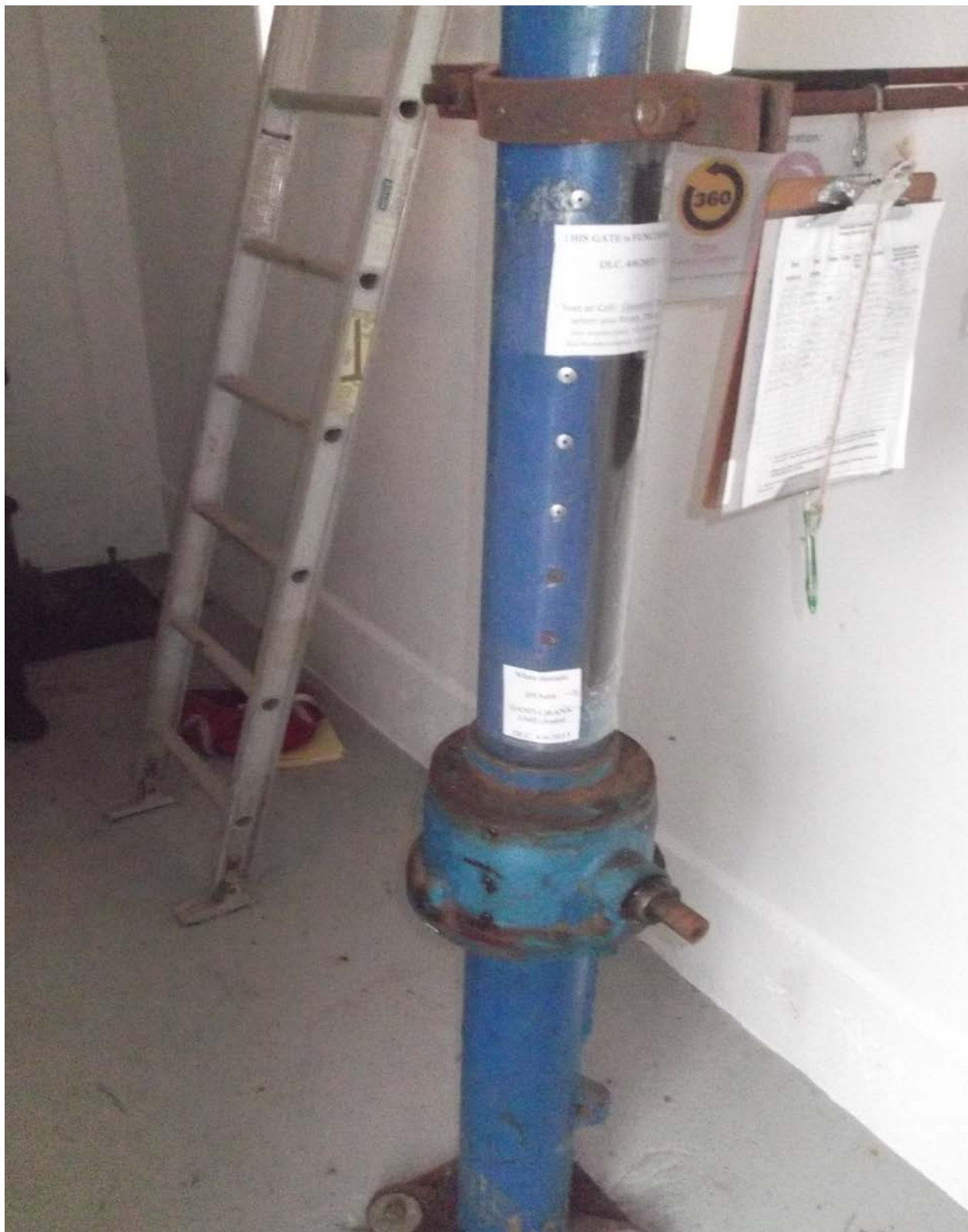
Existing Manual Gate Actuator to be Motorized- Two of Two
