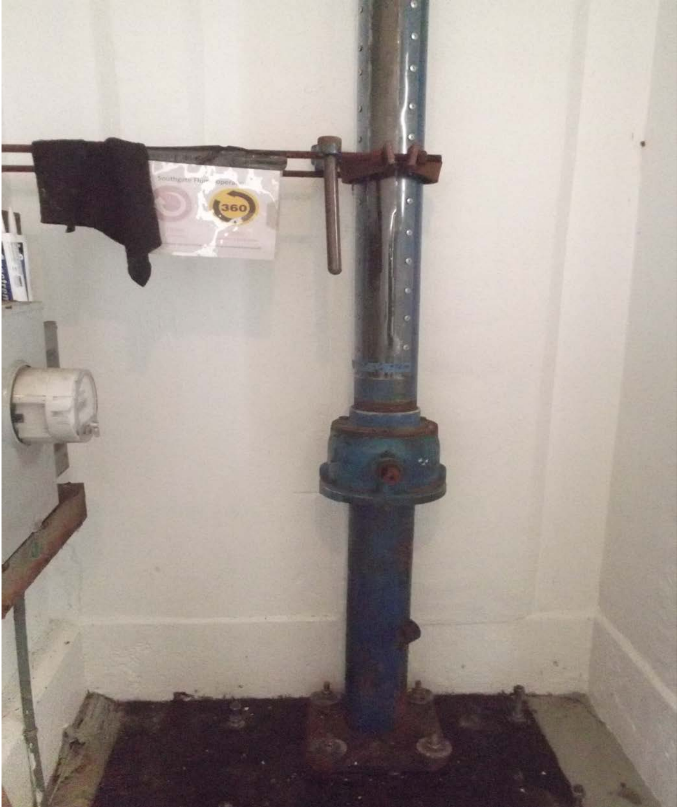
Existing Manual Gate Actuator to be Motorized – One of Two
